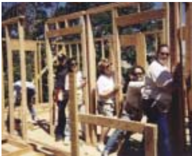
San Leandro employees volunteered for two days to work on a new house in Crockett, California, for Habitat for Humanity.
