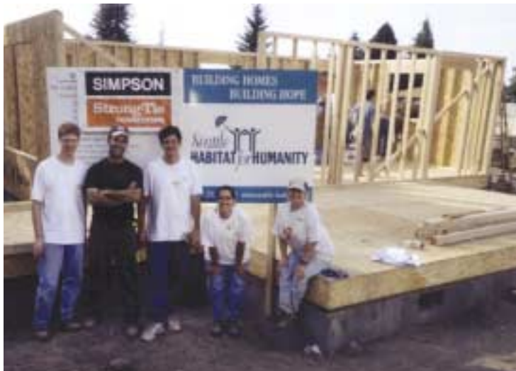
A San Leandro, California, employee volunteered time to help install structural connectors in 10 Habitat for Humanity homes in White Center, Seattle Washington.
